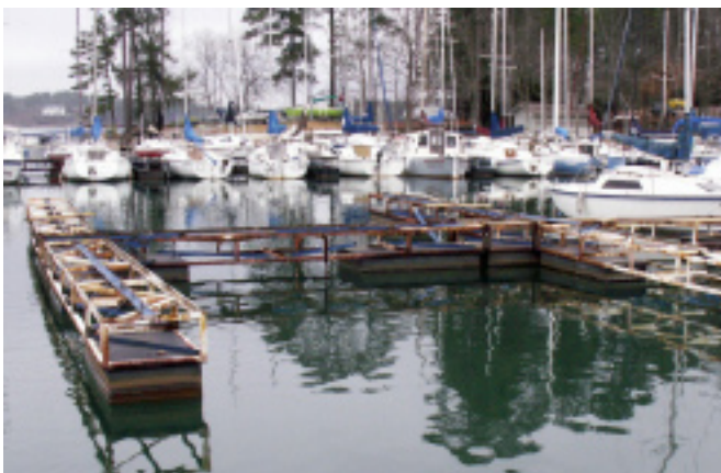
End Section, Dock 2, Decking Gone
